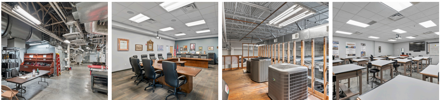
Sheet Metal Workers Local 36 replaced old fluorescent lamps with Keystone LED lamps. The upgrade is helping simplify maintenance and save energy, supporting the building's LEED-certified status and providing a more welcoming atmosphere to its many visitors and employees.
